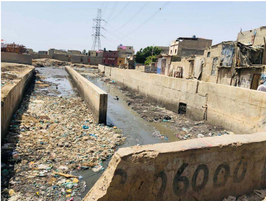
Figure 8: Failed government-executed infrastructure
