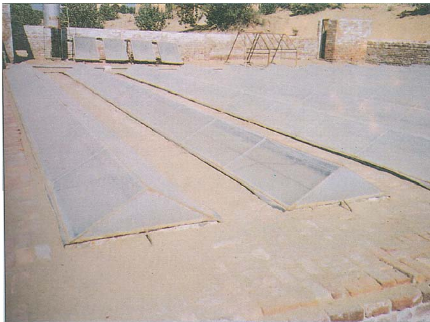
SAZDA installed desalination plant at Vajoto
