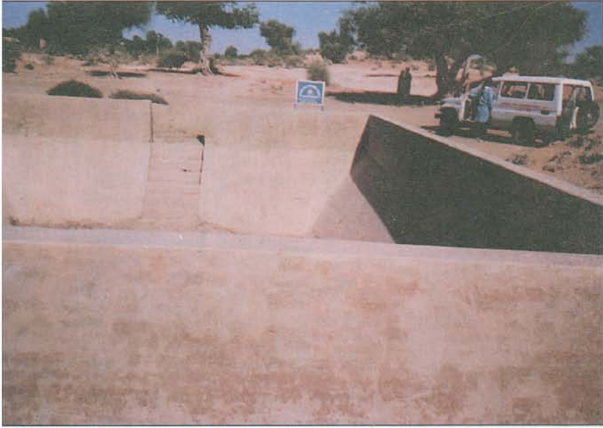
Waste water problems at SAZDA water supply tanks
